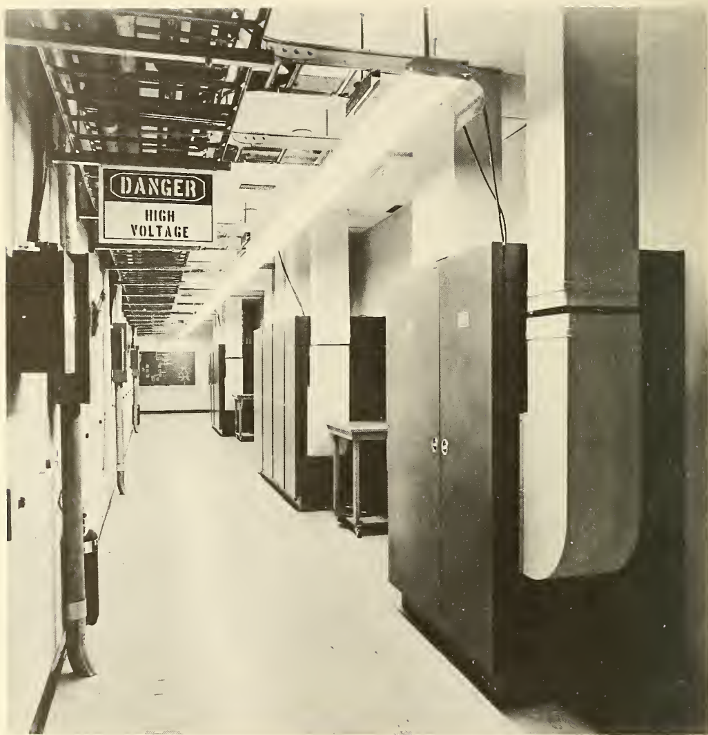
Figure 7. The south corridor of the building behind the transmitters, showing overhead cable trays, power line disconnect switch, and air ducts to the transmitters.
